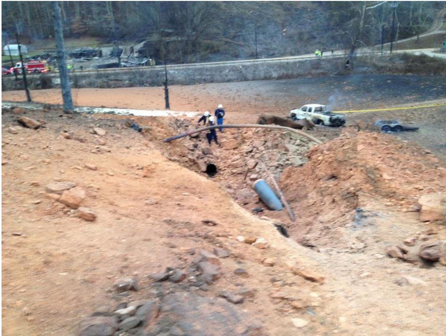
Figure 11- Crater at Sissonville, West Virginia. This is quite typical of a transmission pipeline explosion.
