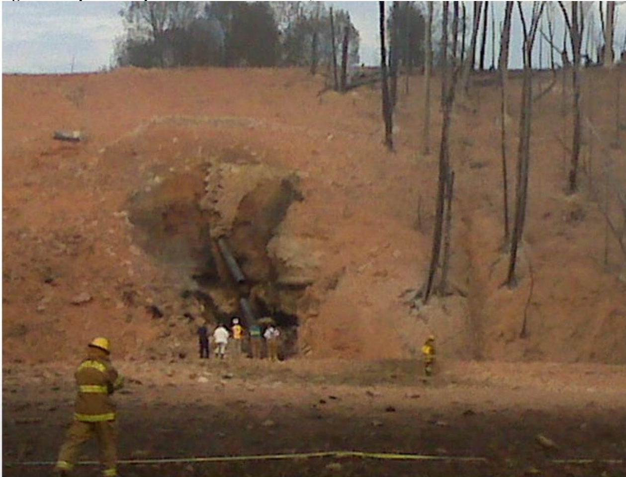
Figure 3- Pipeline Rupture 5/5/2009 Rockville, In Ref 16
