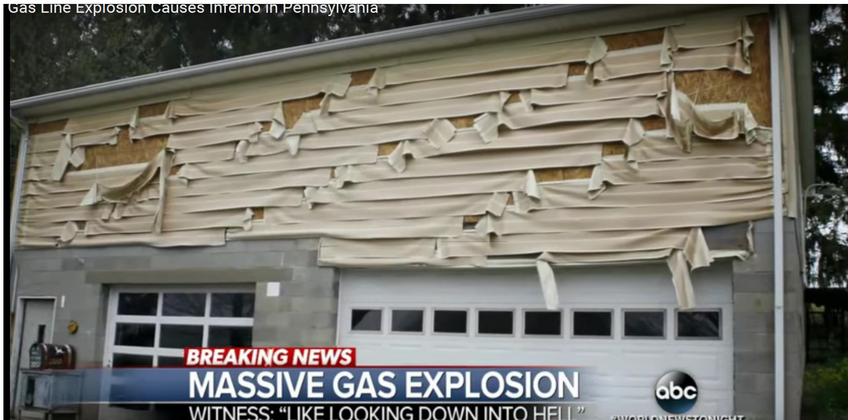
Figure 18 - Sliding melted on house 895 feet from rupture Salem Township, Pa. Ref 19
